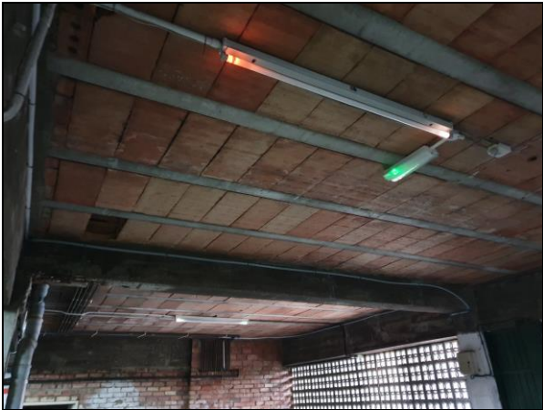
Faulty fluorescent light fittings
